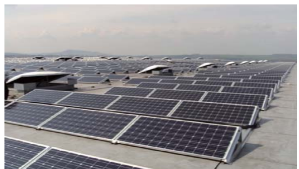
Roof Mounted 1MWp installation
