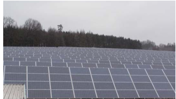
Ground Mounted 10MWp installation
