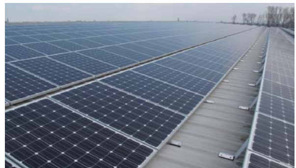
Roof Mounted 2MWp installation
