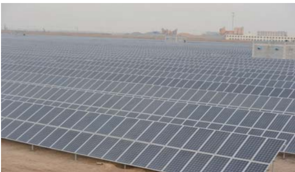
Ground Mounted 7MWp installation
