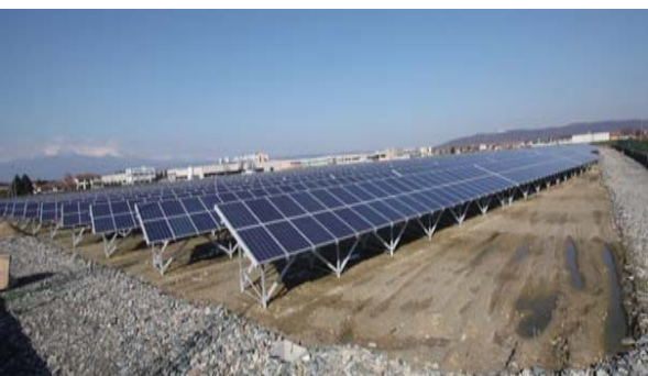
Ground Mounted 2.5MWp installation
